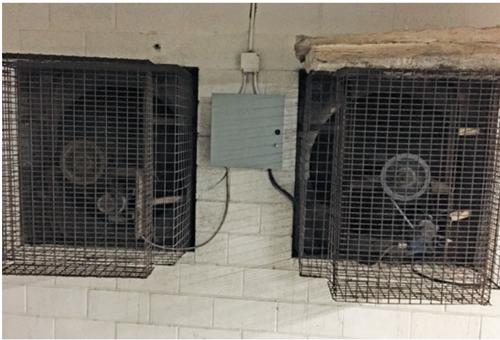
Running garage ventilation fans continuously was adding thousands of dollars annually to the energy bill.
